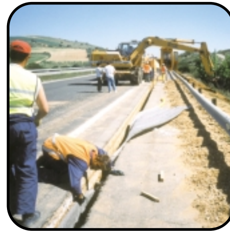
Highway, Spain Road edge drain
